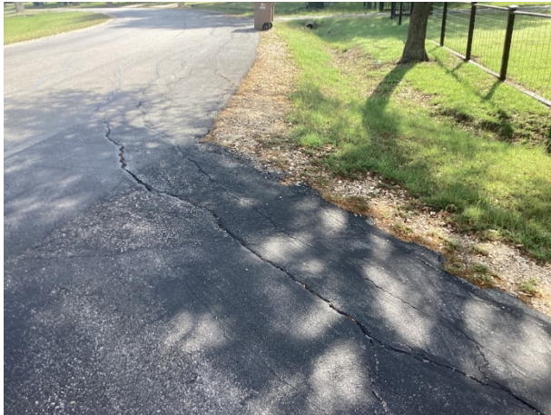
Slippage cracks near park entrance
