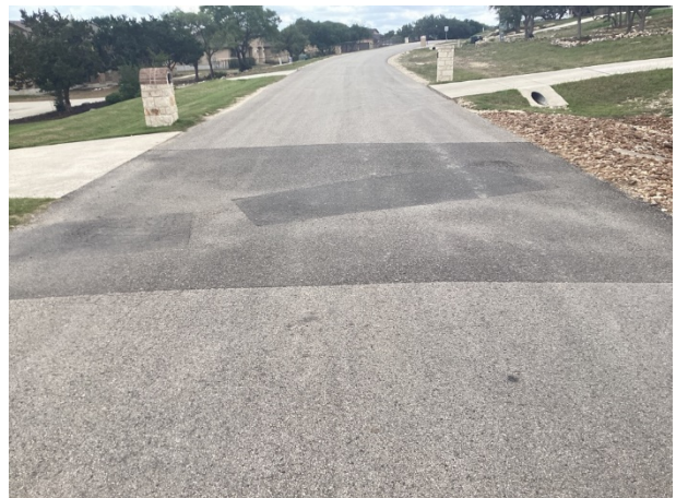
Patch with alligator cracks at Lantana Crossing
