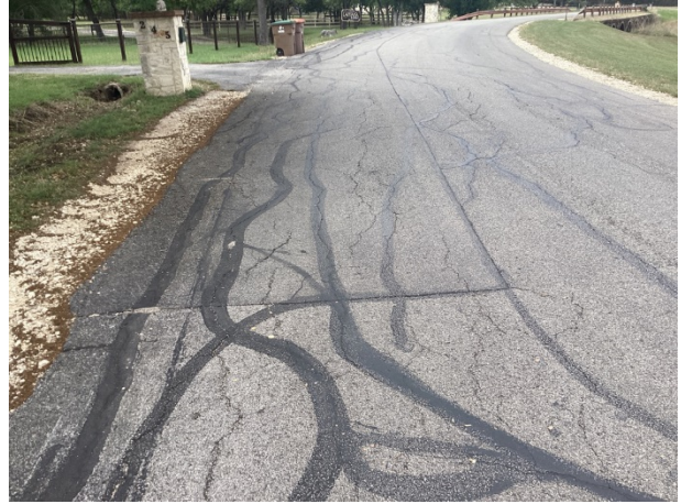
Pavement cracks at Lantana Valley
