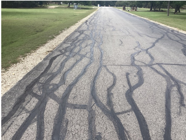
Pavement cracks at Lantana Valley
