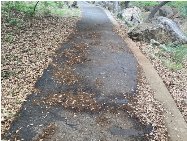
Walking path cracks
