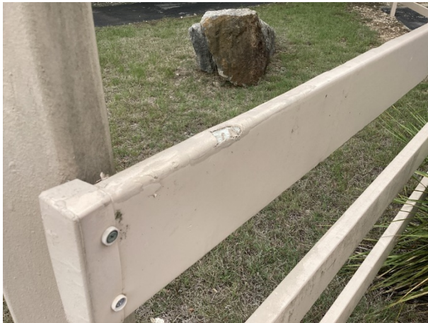
Vinyl wrap deterioration
